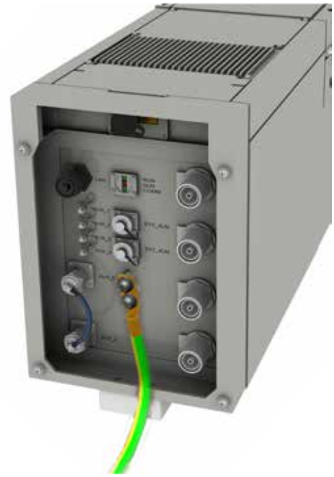
Figure 11. GX Grounding Connection
