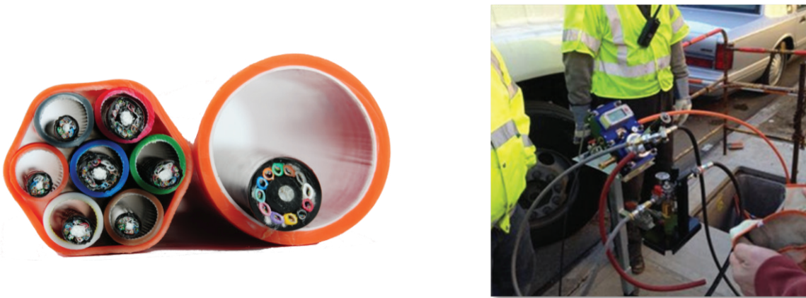
Figure 6. Air Blowing Light-weight Microcables Provides a Fast and Efficient Way of Increasing Transmission Capacity
